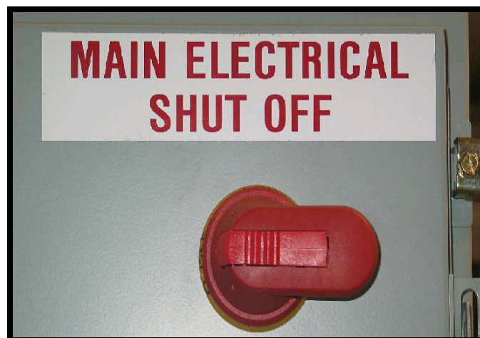
Figure 3. Main Electrical Shut Off Control With Lock Out Tag Out Switch (if applicable).
